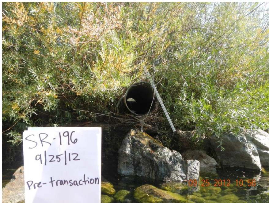
Figure 29: Scott River #196: Fish bypass outflow pipe, before transaction.
