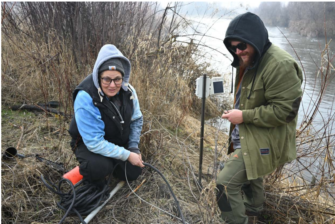
Photo 10: Static staff gage sensor deployment wire protection application connected to remote data transmitter (hard plastic conduit and abrasion resistant soft wire sheathing are used to cover any exposed wiring, in and out of the water). (SRCD, 2025).
